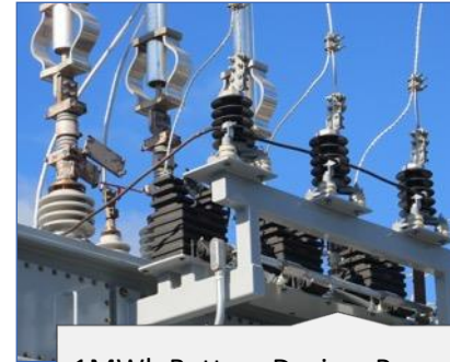
1MWh Battery Design, Proc. and Impl. Cape Verde
